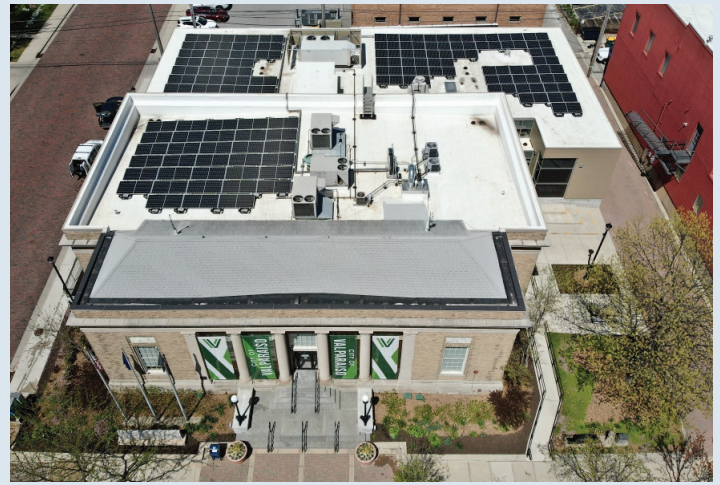
Valpo's sustainable solar project added 772 solar panels to five City facilities, saving taxpayers more than $5.2 million in electrical costs over the life of the panels.
